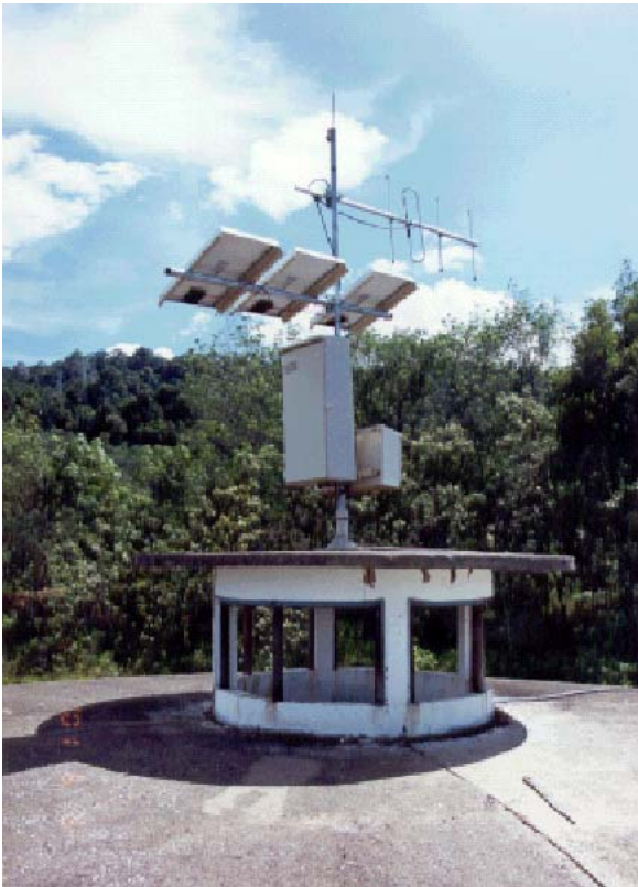
Solar Powered Remote Terminal unit (RTU) installed on top of a reservoir
