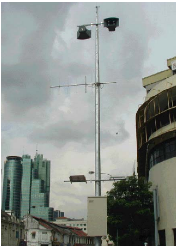
Solar powered early flood warning siren VHF RTU Installation on 12m siren mast
