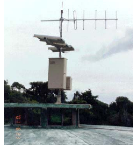
Reservoir level monitoring using telemetry system
