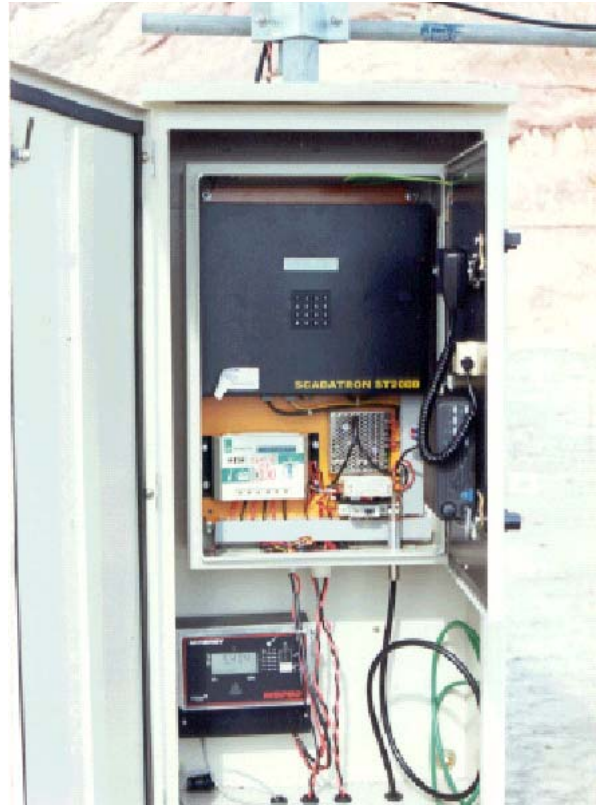
Internal view of the RTU housing shows Controller, radio and ultrasonic sensor
