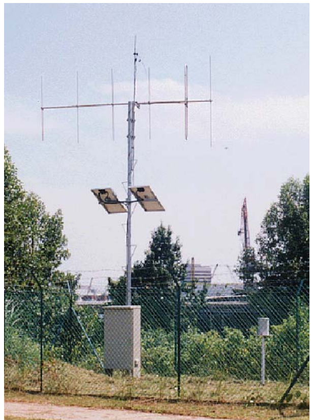
Typical Rainfall Outstation shows RTU Housing, solar panels, antenna and rainfall sensor
